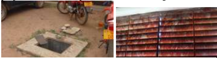
Figure 8 Open manholes at Pader Court and poor ventilation in cells of kaberamaido Police
